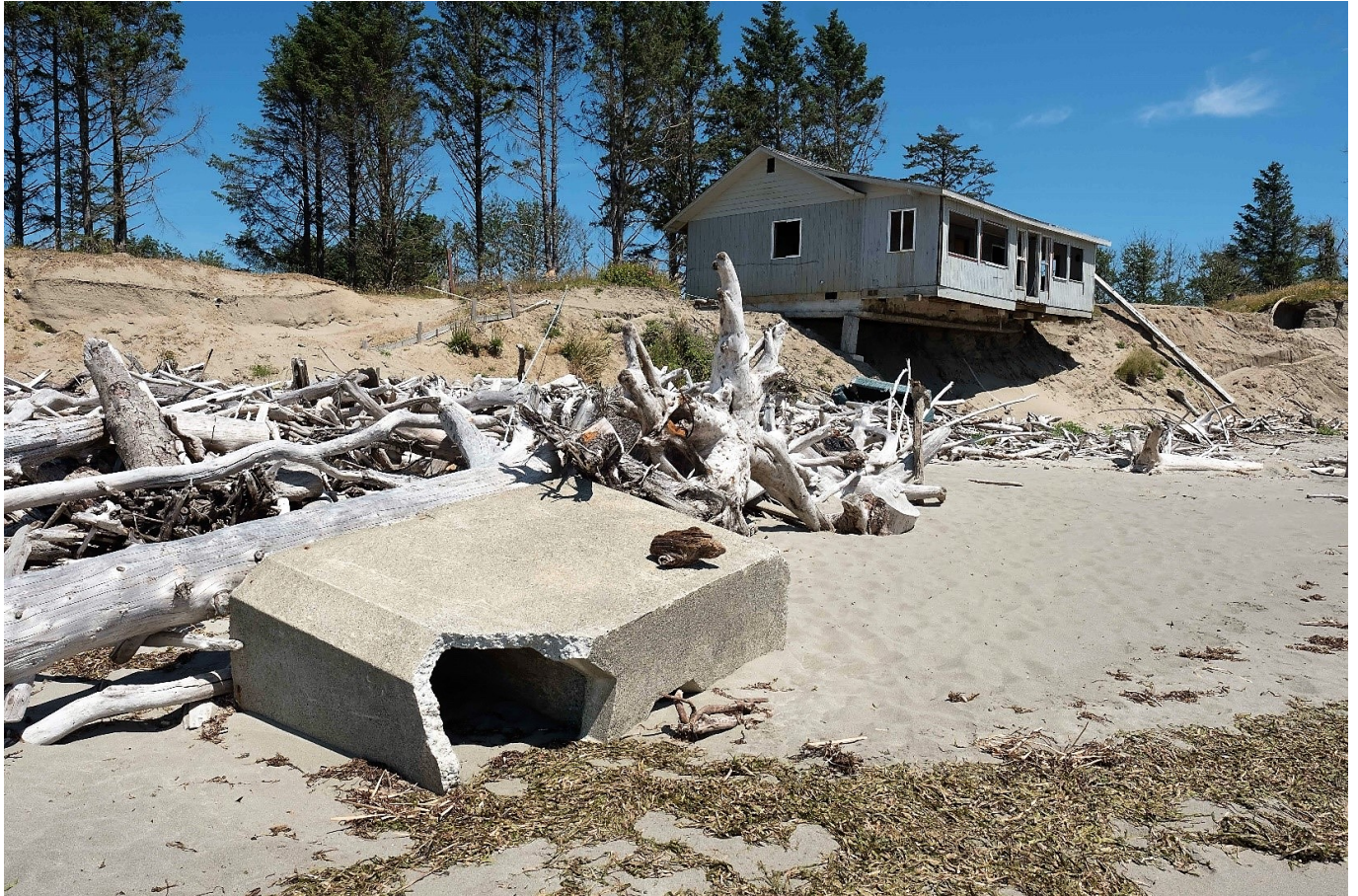
Caption: A home in North Cove, WA that faced significant coastal erosion (source: Kit Swartz).
