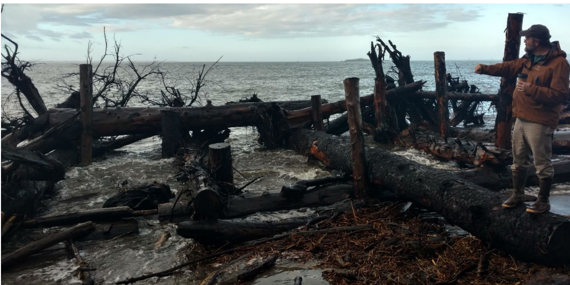
Top left: Scour is evident where water passes through gaps in the structure, making the structure less stable.
