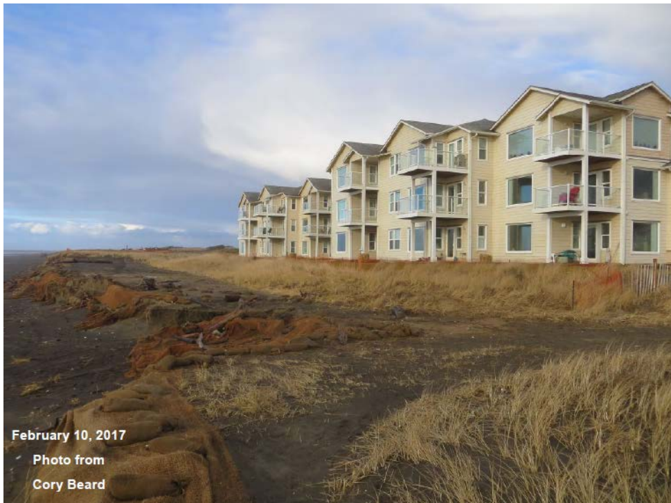
Figure 3-5: Ground-based photograph of emergency protection measures and coir mat on the seaward face of the erosion scarp
