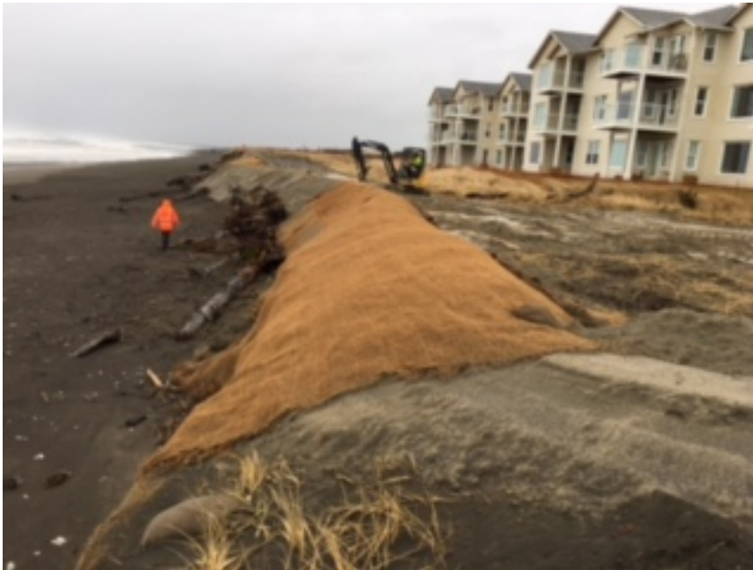
Figure 3-7: Ground-based photograph of emergency protection measures and coir mat on dune face with repairs in progress (photo taken February 15, 2017 by Robert Parnell)
