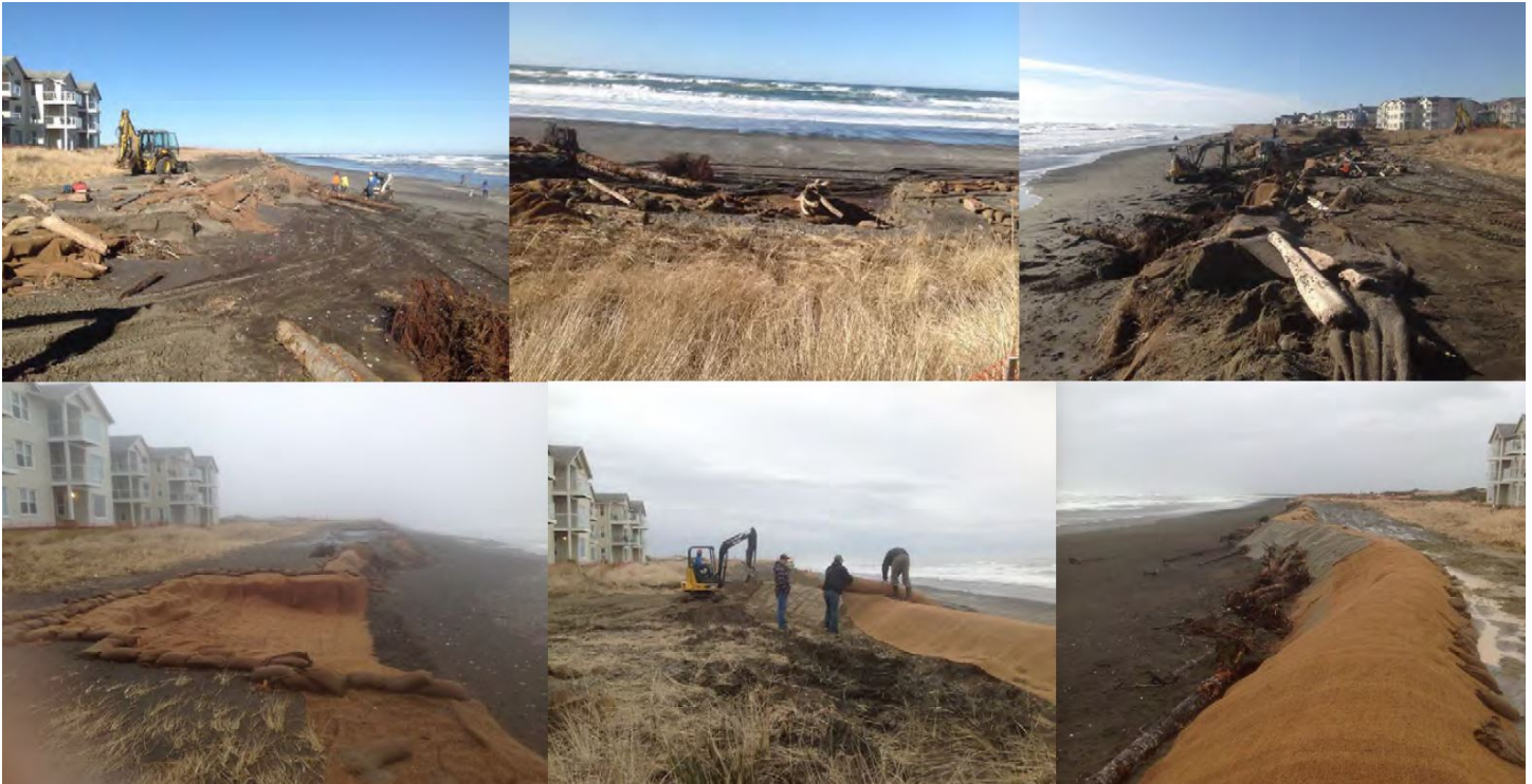
Emergency protection measures with coir mat on the seaward face of the eroding dune, 2017. Sand had been placed atop coir mat and straw bales in 2016. (Image credit: 2018 Homeowners Associations presentation to Washington State Department of Ecology)
