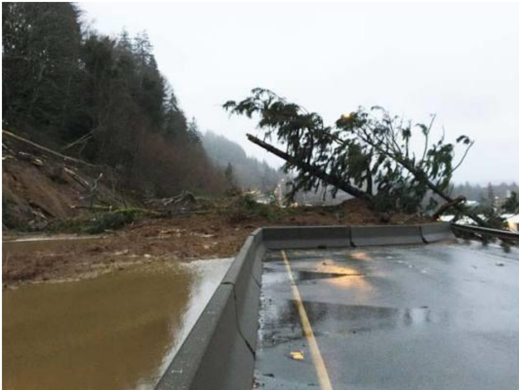
Landslide along Highway 12 in Aberdeen (source: MyNorthwest.com)
