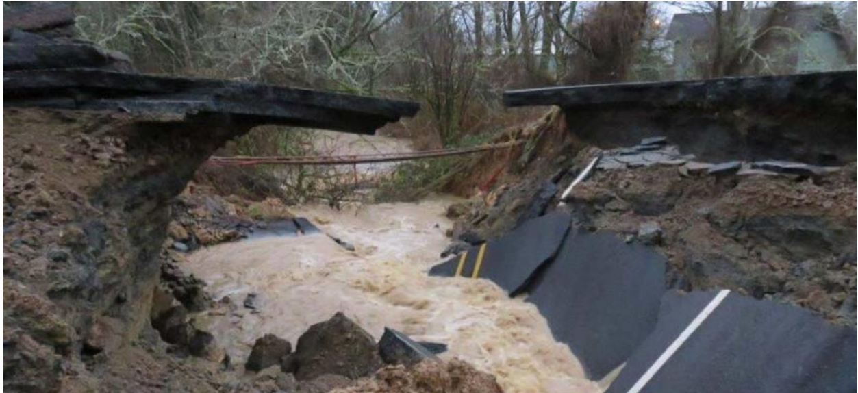
SR 4 west of Naselle is closed between US 101 & SR 401 due to a collapsed culvert (source: mynorthwest.com).
