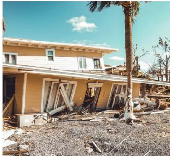
Damage caused by Hurricane Michael in Mexico Beach, FL
