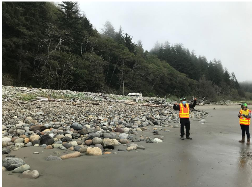
Figure 1. WSDOT staff stand in front of a pilot dynamic revetment installed in front of SR 105 on the western side of the project site area, 2020.
